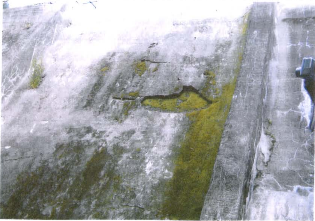
Photo 2 ID# 230-0677 Harlem Valley State Hospital Res Dam 6/28/07 Downstream face of the spillway
