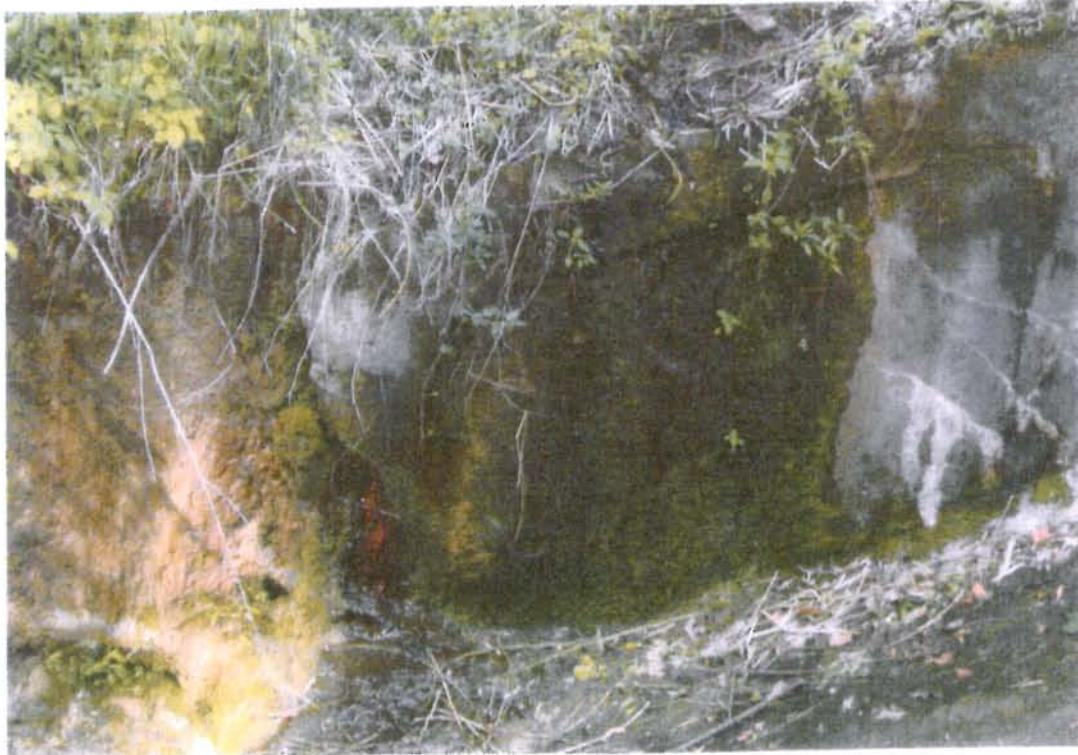
Photo 4 ID# 230-0677 Harlem Valley State Hospital Res Dam 6/28/07 Seepage through right wall
