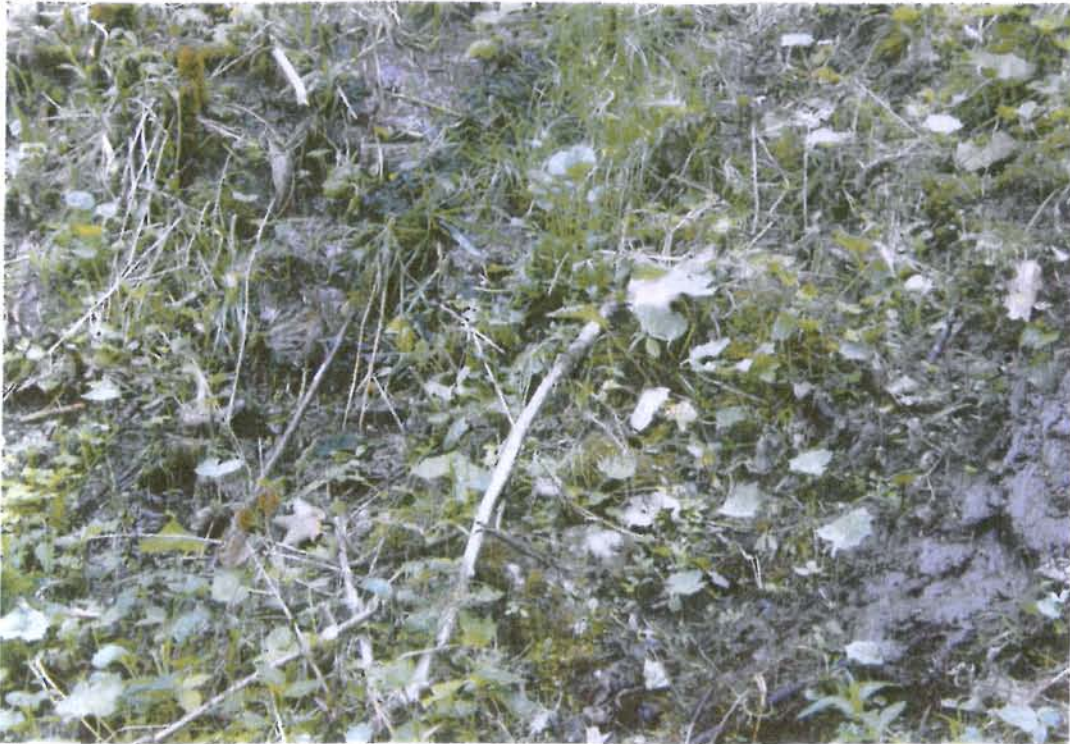
Photo 5 ID# 230-0677 Harlem Valley State Hospital Res Dam 6/28/07 Wet area downstream - left of spillway
