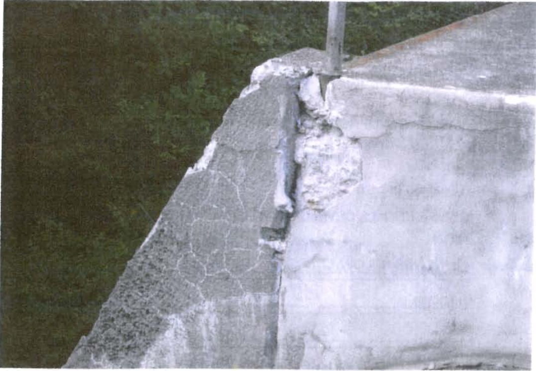
Photo 1 ID# 230-0677 Harlem Valley State Hospital Res Dam 6/28/07 Concrete spalling on right spillway wall
