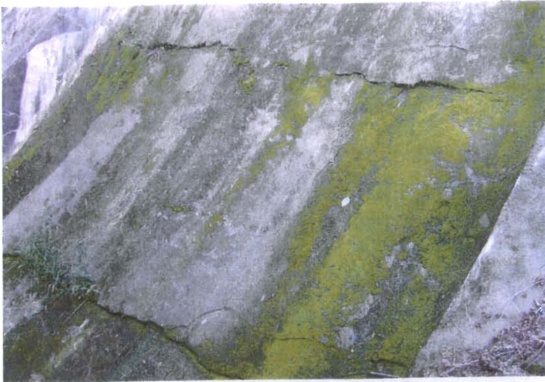
Photo 3 ID# 230-0677 Harlem Valley State Hospital Res Dam 6/28/07 Horizontal cracks - downstream face of dam
